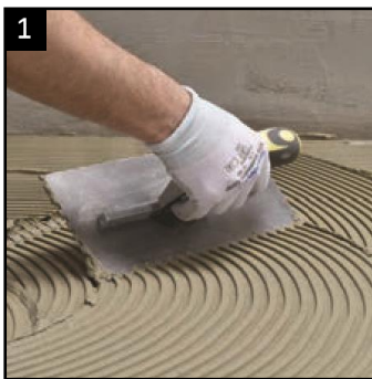
1 Spread tile adhesive Spread a flexible cement based tile adhesive over the floor.
