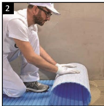
2 Lay the membrane Roll the membrane out over the whole floor and press into the adhesive.
